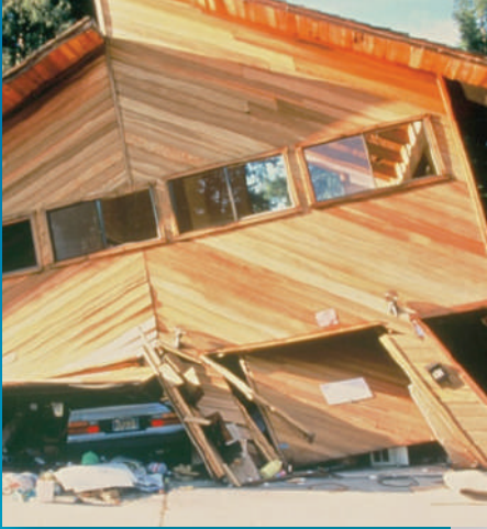
The walls around the garage door of this home were not strong enough to withstand the shaking of the 1989 Loma Prieta Earthquake.
